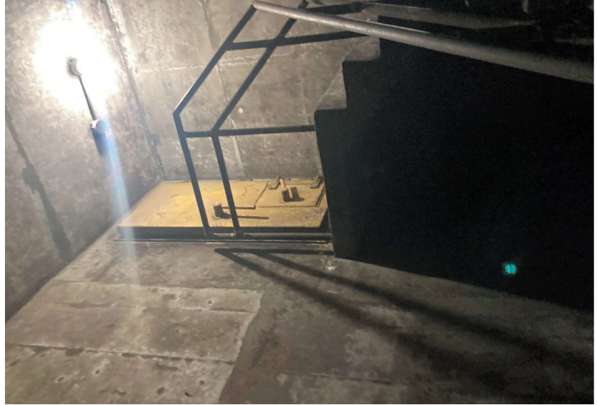
View from entry way after entering stairwell from roadway looking up at plenum access door.
